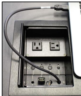
Figure 10 - Connecting a Laptop Using HDMI Supplied by Instructor Station
